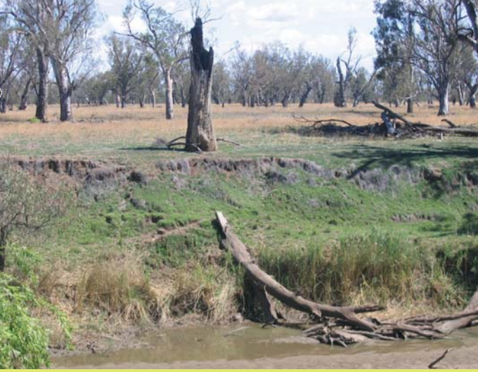
Comparisons between the fenced river bank on Vic Melbourne's side (no lippia) with the unfenced bank directly across the river. Uncontrolled cattle access has resulted in increased lippia, leading to bank slumping
