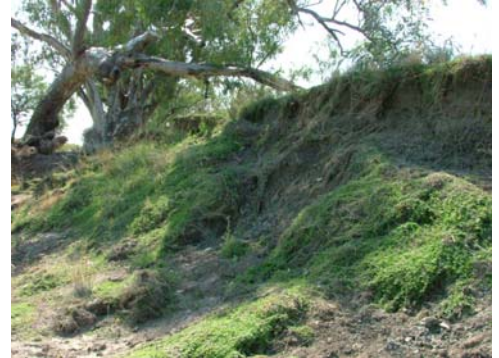
Above: Slumping and erosion in Croppa Creek, which runs through the Gooderham's property.
