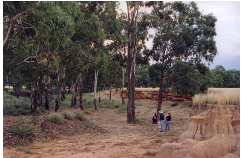
A rock groyne was placed in the creek to divert flows and minimise erosion.
