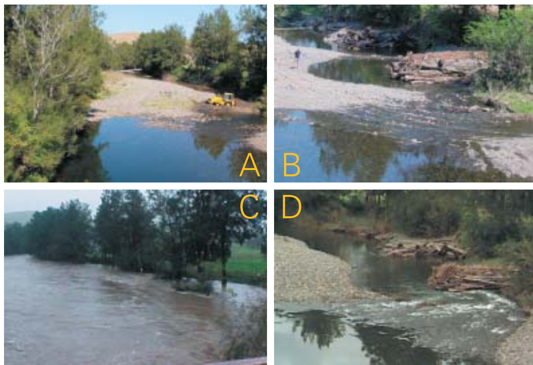
These photos (A–D) show the construction of an engineered log jam that is designed to increase aquatic habitat and diversity in the river channel. Even after the large flood shown in Photo C the log jam remained in place, with Photo D showing how the log jam structure is changing the river channel to create a range of different habitats for plants and animals. Williams River, NSW. Photos Andrew Brooks.
