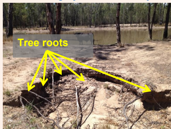
Figure 5: Tree roots and debris build up contributes to gully erosion in dam bywash
